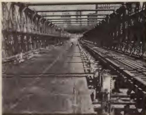
The intermediate truss completely removed, the outer truss in position and overhead struts all in place, old roadway untouched as yet.
